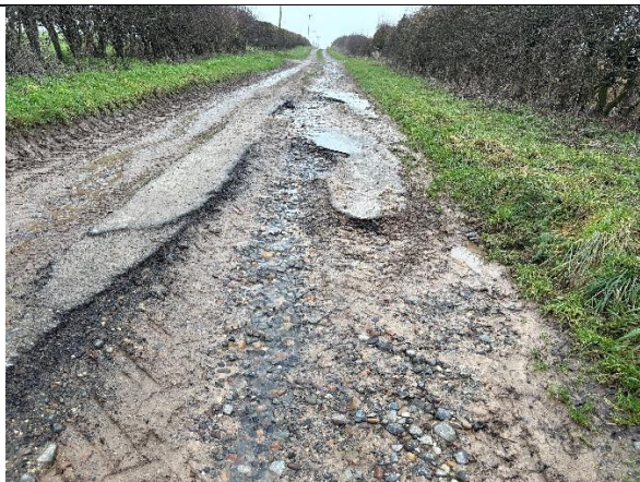
Figure 1.4 Signs of Previous Pavement
