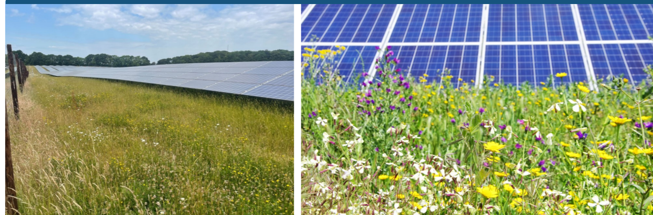
Example Ground Mount Arrays
