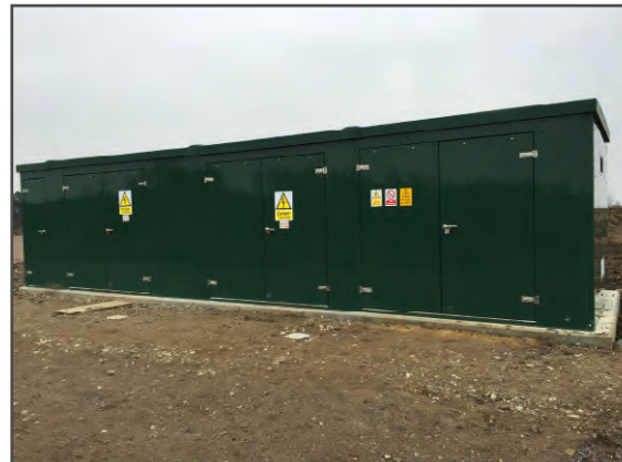
Plate 7.9 - Typical Brick and GRP Substation Units
