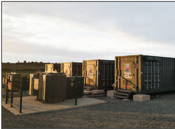
Plate 7.7 - Typical Battery Energy Storage System
