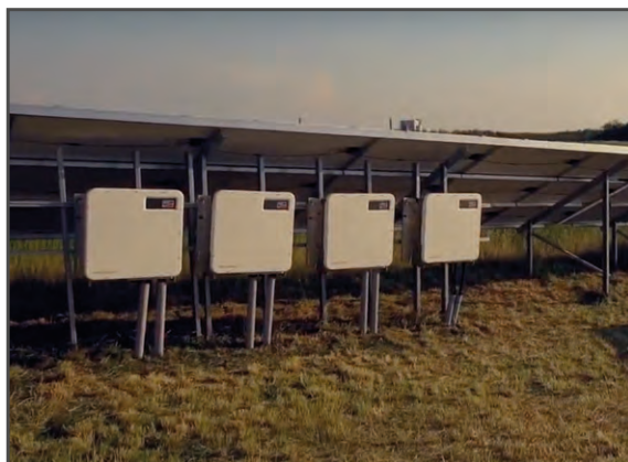
Plate 7.3 - Typical string-inverter units
