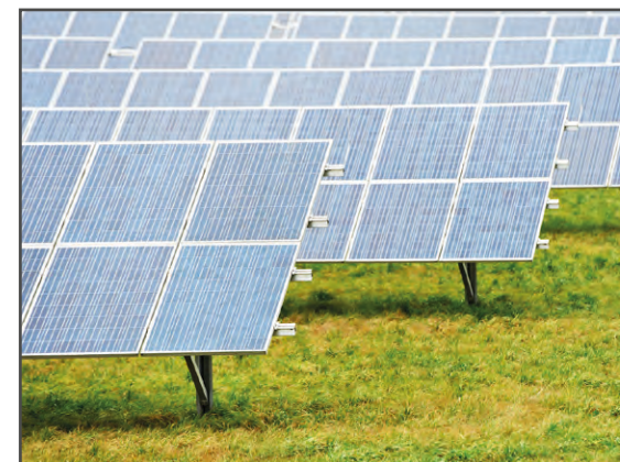
Plate 7.1 - Typical Ground-Mounted Solar Array on Frame
