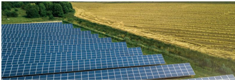
Rows of solar panels
